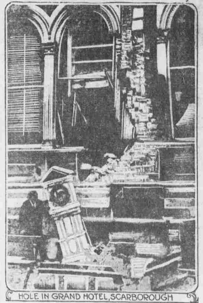
HOLE IN GRAND HOTEL, SCARBOROUGH
