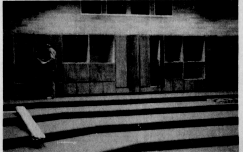
MUSIC ROOMS situated in the back part of the Auditorium are nearing completion. The band room, above, occupies one end of the building. A similar chorus room is on the other side, with offices, storage and practice
