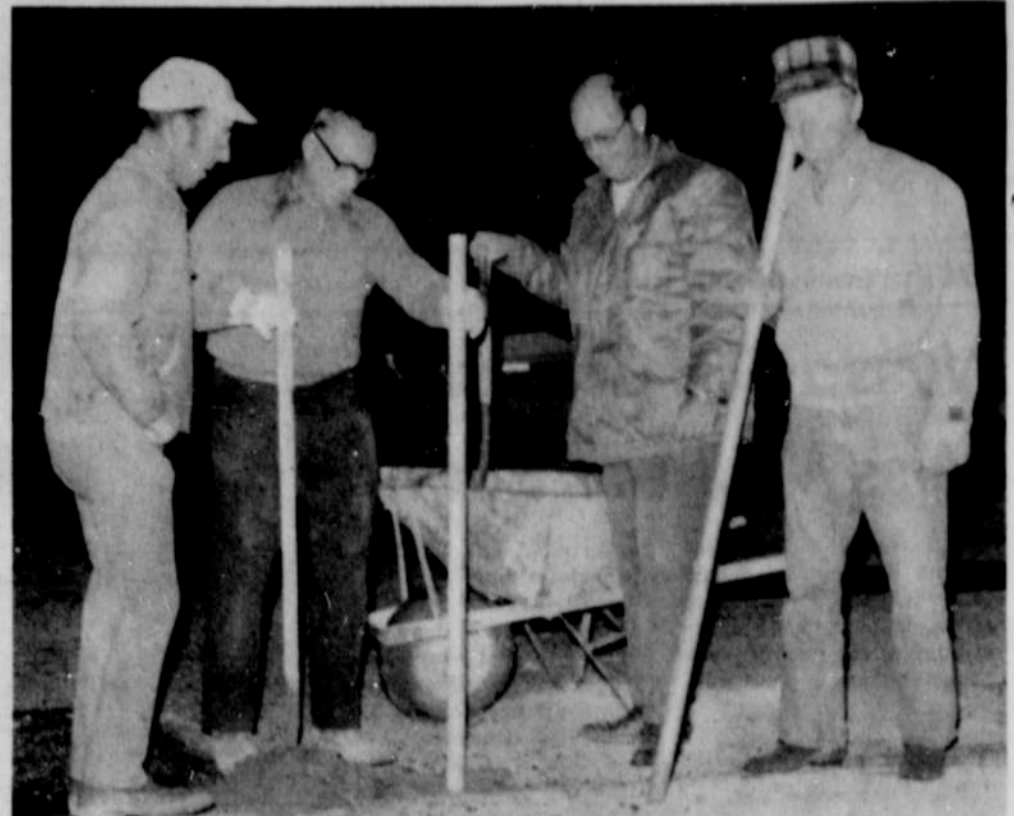
GROUND WORK FOR A FENCE around the nursing home was started several days ago. The fence is being erected by volunteer workers and it is a project of the Malheur Memorial Hospital Auxiliary Workers
