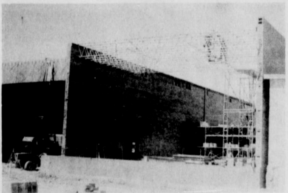
TRUSS-JOIST BEAMS are being installed in the new gym, with the huge laminated beams over the playing floor visible at left.
