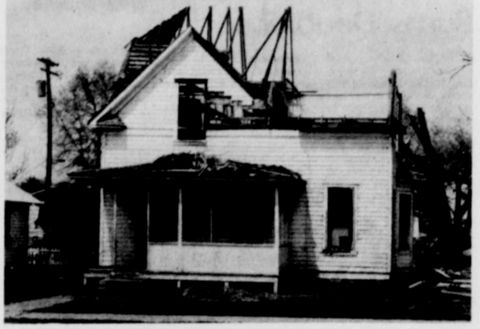
ANOTHER OLD LANDMARK, this house at 214 Ehrgood, is being torn down. The work is being done by Joe Costello, Arthur Harris and families.
