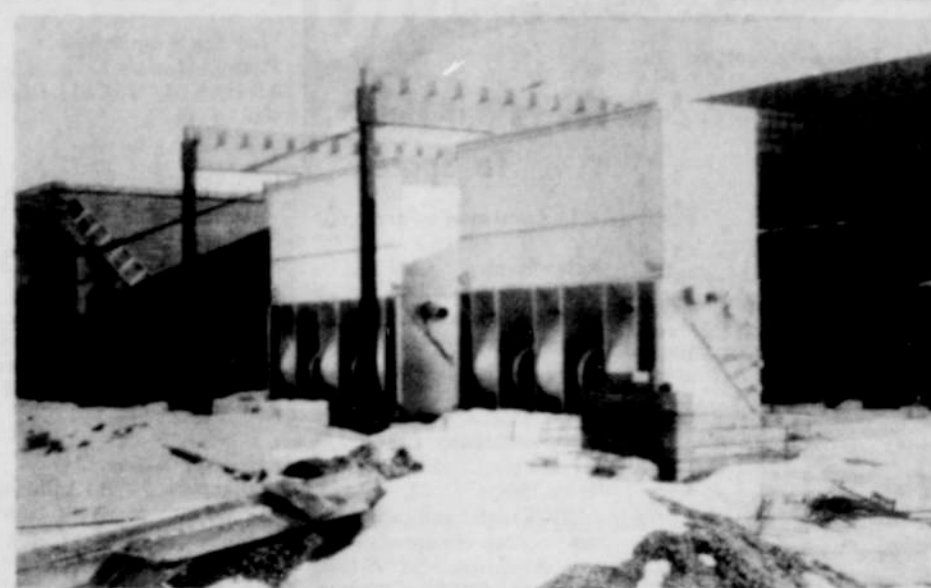
COOLING TOWERS HAVE BEEN INSTALLED in the mechanical building for the Nyssa Schools. When all the machinery has been installed the walls and roof will be completed.
