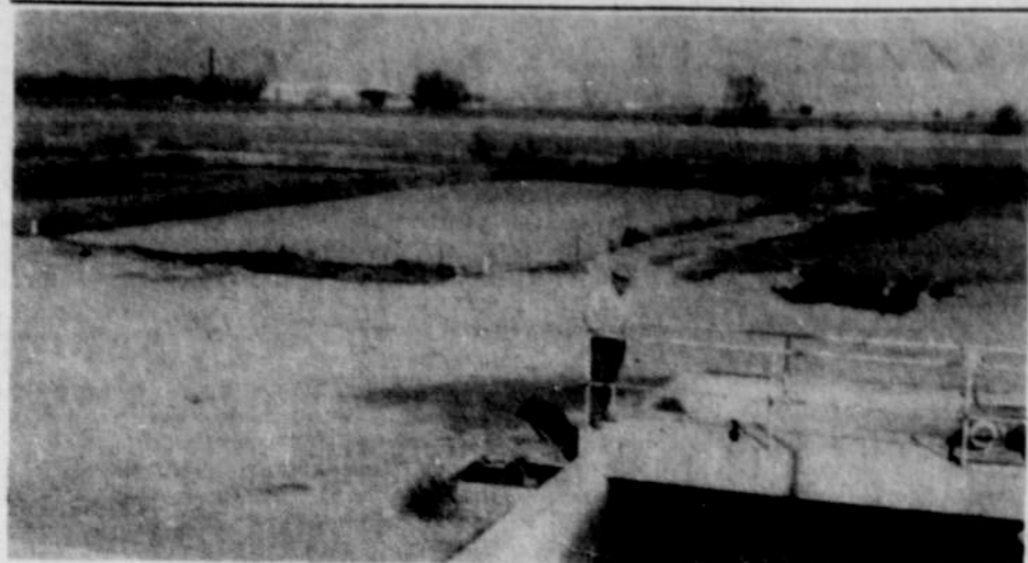
SETTLING PONDS FOR SEWAGE SLUDGE are pictured at the Nyssa Sewage Disposal Plant, with Plant Operator Frank Lawrence standing on the catwalk. City crews have
