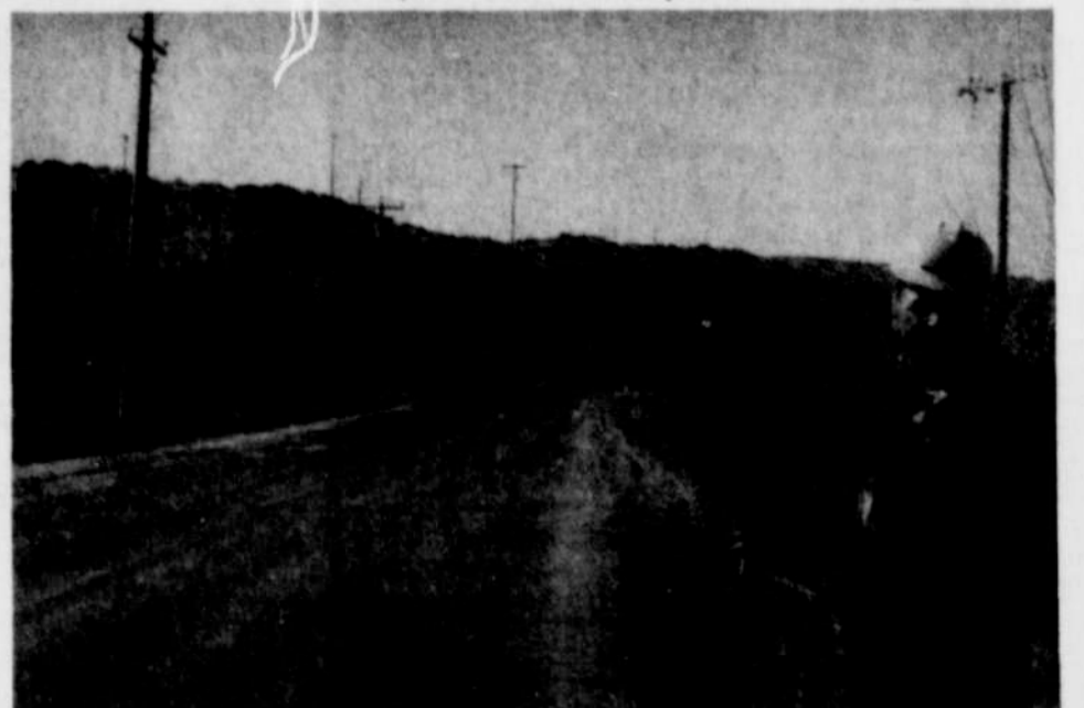
THE STATE HIGHWAY DEPARTMENT is widening State Highway 201 between Owyhee Junction and Adrian. This picture taken Tuesday shows the crews working in
