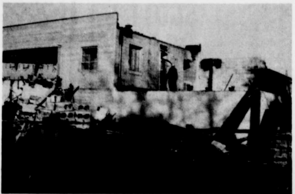
DEMOLITION OF THE OLD FIRST National Bank Building is underway, with most of the building gutted on the inside, and the walls expected to topple later this week. The wall remaining in the background belongs to Brackens Department Store.
