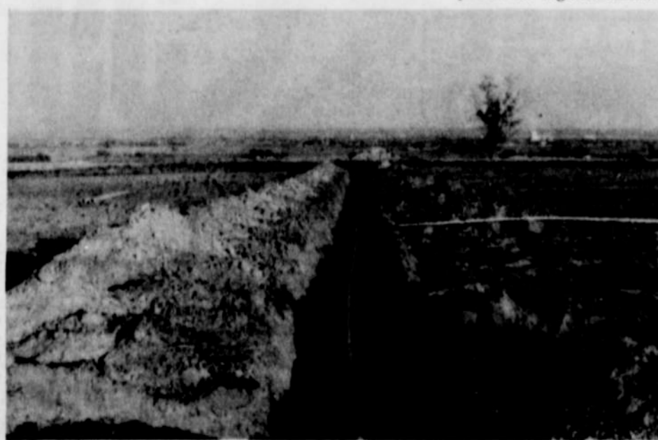
CITY CREWS ARE INSTALLING a pipeline and preparing to seed a section on the east side of the Nyssa Cemetery. An 815-foot roadway will encircle this section, and planting will get underway as soon as the sprinkling system is installed in the area on the right of the photo.
