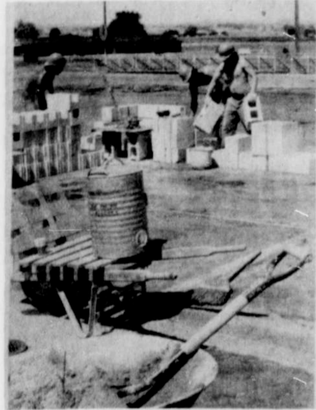
THE MARSING JOB CORPS started work on the rebuilding of the Nyssa school shower facility last week and have begun erecting the walls of block brick. Director of the operation is Weldon Fisher who is brick laying instructor for the Marsing Job Corps. He said the young men working on the building are working toward apprenticeships in the Bricklayers International Union.
