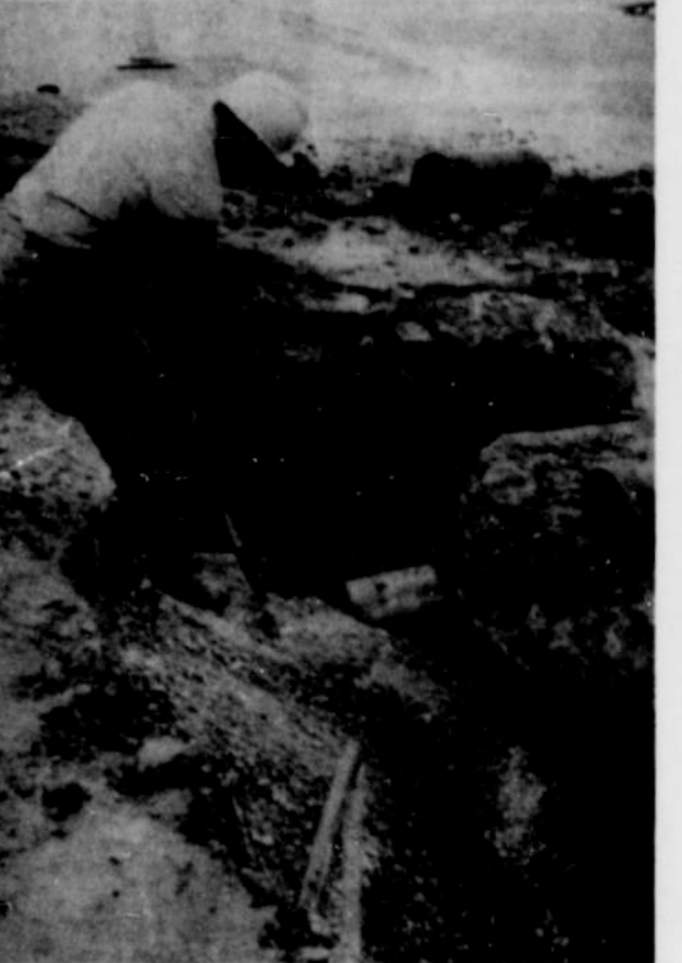
DEAN WINCHESTER WORKS in the hole last Monday at the intersection of Main and South First Streets in Nyssa. A water main broke early Monday morning at 3 a.m. and water was turned off to about a two block area in downtown Nyssa for six hours until the repair was completed at 9 a.m. by Water Department Supervisor Ralph Lowe. After the broken pipe was replaced, Winchester and co-workers of the City's Street Department got the chore of filling in the hole.
