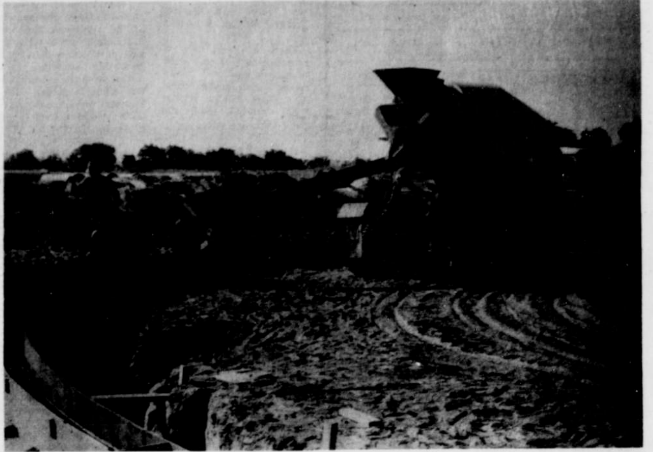
The pouring of concrete for the four-foot high foundation ring wall is shown here as work continues in the readying of Airport Hill for a three-million gallon water storage tank. The new water tank, expected to be completed by August 1975, will increase Nyssa's water storage capacity by 20 times the existing capacity. Nyssa is able to hold 150,000 gallons now.
