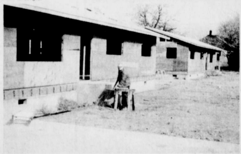
SELF-HELP HOUSES UNDER CONSTRUCTION between 1st and 2nd Streets on Ehrgood Avenue will receive help from the Building Trades class of Nyssa High School, under the supervision of George Fanning, shown above.
