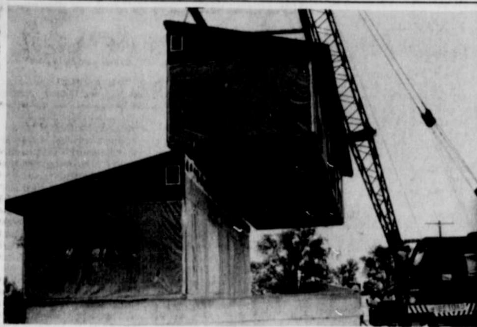
THE NEW HOME OF MR. AND MRS. HARVEY Wilmot took shape in a hurry last Friday as Boise Cascade crews brought in the pre-built components and lowered the two 30,000 pound sections onto the daylight base-ment. The new house is being built in the 800 block on Bower, just north of the Nyssa Elementary School playground.
