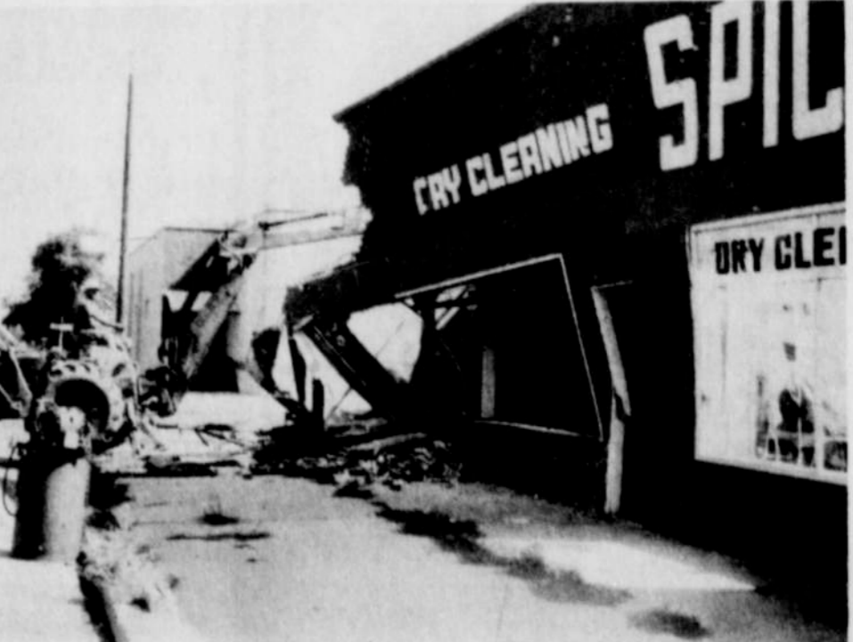
THE SPIC & SPAN CLEANERS, owned by Mr. and Mrs. Jim Tomjack, is rapidly being demolished to make way for a new modern building on the same corner of 3rd & Bower. The business was destroyed by fire the evening of June 10.
