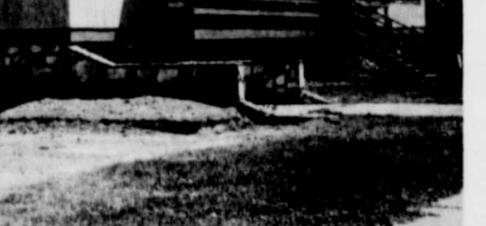
THIS FINE NEW APARTMENT HOUSE is nearing completion on the corner of 3rd Street and Park Avenue. Built on the old St. Bridget's Parish Hall basement by Dale Schraufnagel and Deryl Leggett, Nyssa High School teachers, the apartment is a fine and needed addition to the city.
