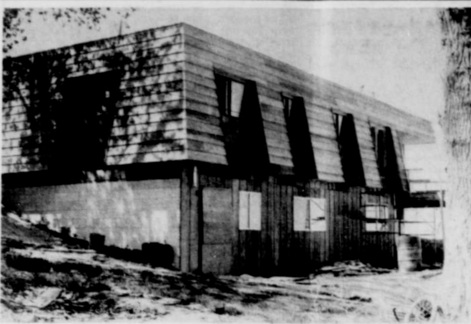
ANOTHER FINE NEW HOME nearing completion in Nyssa, this one being built for Mr. and Mrs. Rod Cowgill high on a hill overlooking the valley. This 3,000 square
