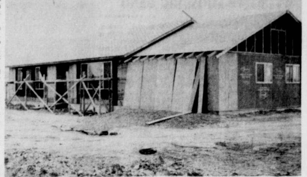
THE NEW HOUSE BEING BUILT by boys in the Building Trades class at Nyssa High School at 11th and Ebgood is rapidly taking shape. Electricity and plumbing has been installed and ready for finishing. The project is under the direction of Bill Hood.
