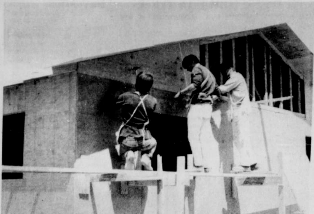
John Marquez, Eloy Diaz, and their instructor, Bill Hood, are shown working on the new home of Rev. David Martinez on North 7th Street.
