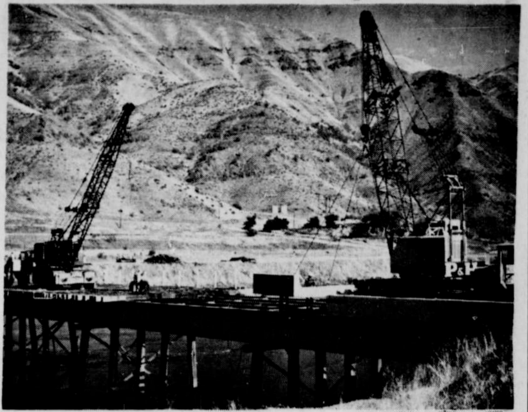
Crane lowers precast slab into position for new concrete deck Idaho Power Company is installing to replace original timber surface on bridge built across Snake River below Brownlee Dam in 1955. New deck, estimated to cost $180,000, is scheduled for completion about October 1. Bridge is one of two the utility built for public access in the T.E. Svach Hells Canyon development.
