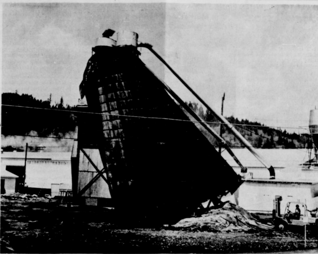
Crrrunch went this Georgia-Pacific "wigwam" waste burner at Yarnell, Ore., plywood plant as it crashed to the ground recently. It is just one of many burners the company is tearing down in its fight against pollution. Material
