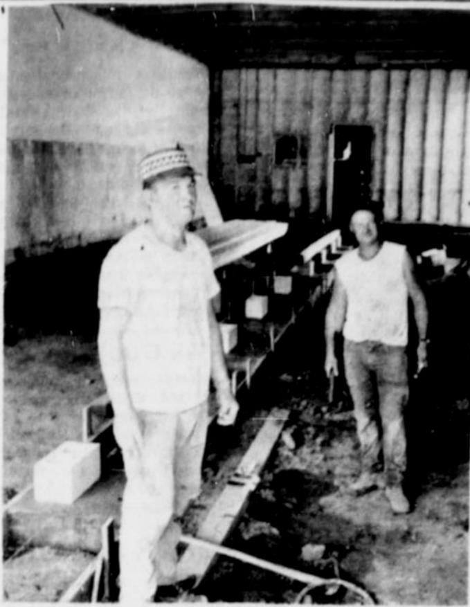
Remodeling is underway on another Nyssa commercial building. Shown here are Rodney Holcomb (front) and Bud Sappe, part of Holcomb Construction crew who are preparing to lay a new floor in the Henigson-Stunz building at 108 Main Street. The front and interior will be remodeled to make office room for the three attorneys and secretaries. It will also include a library common to all three offices. Bob Smith is the architect.
