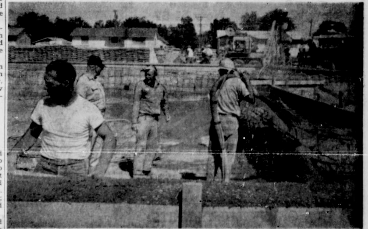
WORK ON NYSSA'S new swimming pool is progressing on schedule and should be completed around the first week in August, according to Art Colby, city manager and resident engineer. Workmen (in above photo, left to right) are Lamar Carlson, roddman; Colby; Dick Allbright, gunite foreman; and Jeff Marchant, gunite nozzleman. To the left is a 500 CFM compressor and air-placo gun being operated by Don Bjerraarde at the swimming pool site, Park avenue, between Seventh and Eighth streets. This equipment can be seen, together with numerous sacks of cement, in the background of the above photo. —Journal Photos.
