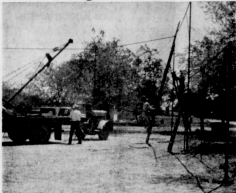
LATEST ADDITION to Nyssa north park is the above newly constructed backstop built solely by donated time and effort as a part of the Baseball for Kids effort. Pictured are Del Malloy, Red McCready and Clarence Lancaster.
