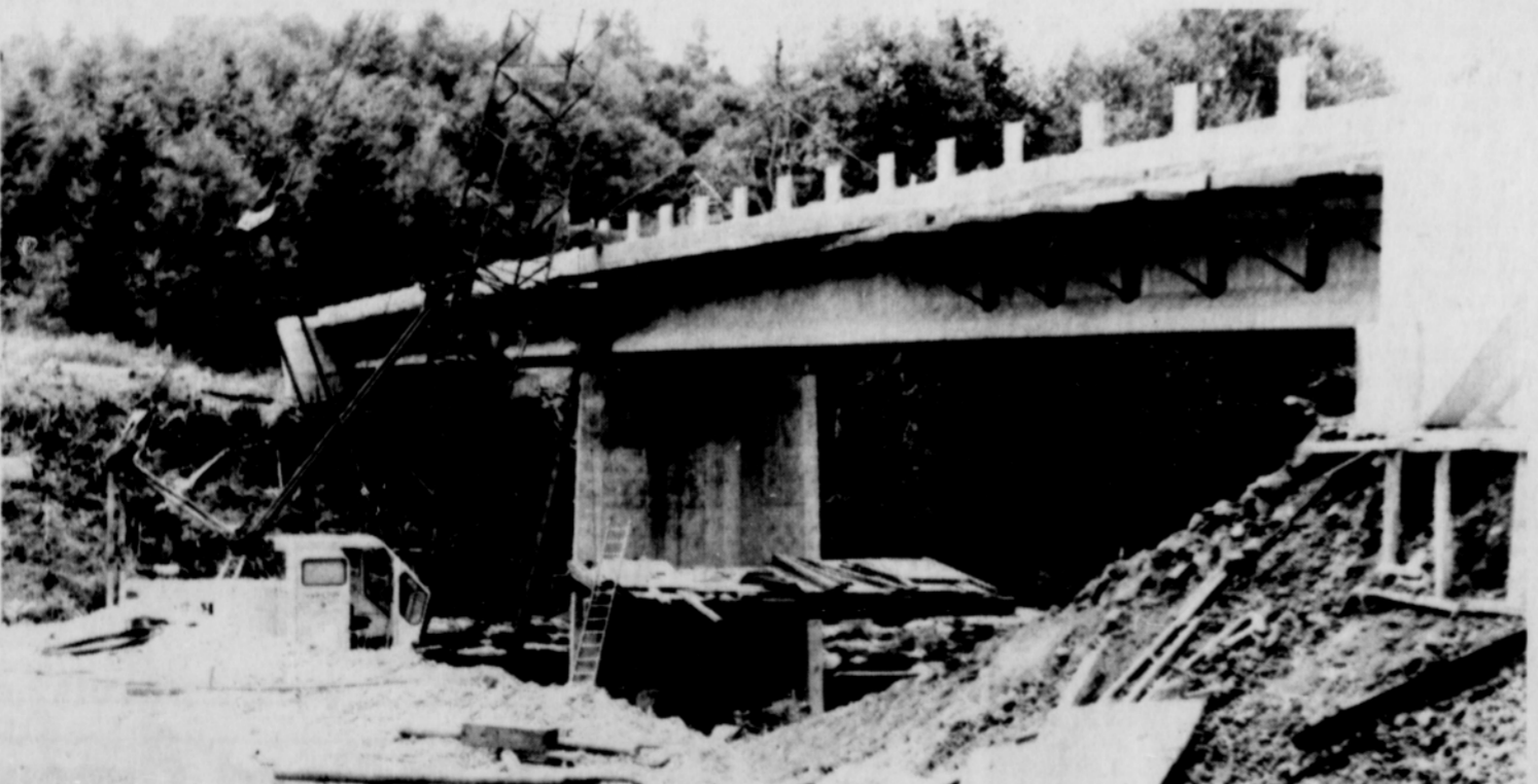
CONSTRUCTION continues on the new bridge being built approximately a quarter of a mile past the town of Mist, replacing the one severely damaged in the January flood. Work on the
