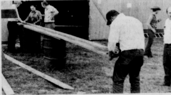
ABOVE, Columbia County Fair Board members are shown cutting cross braces to shore up a building at the County Fairgrounds ruled unsafe for occupancy by Columbia County Building Inspector Ron Eshelby.
