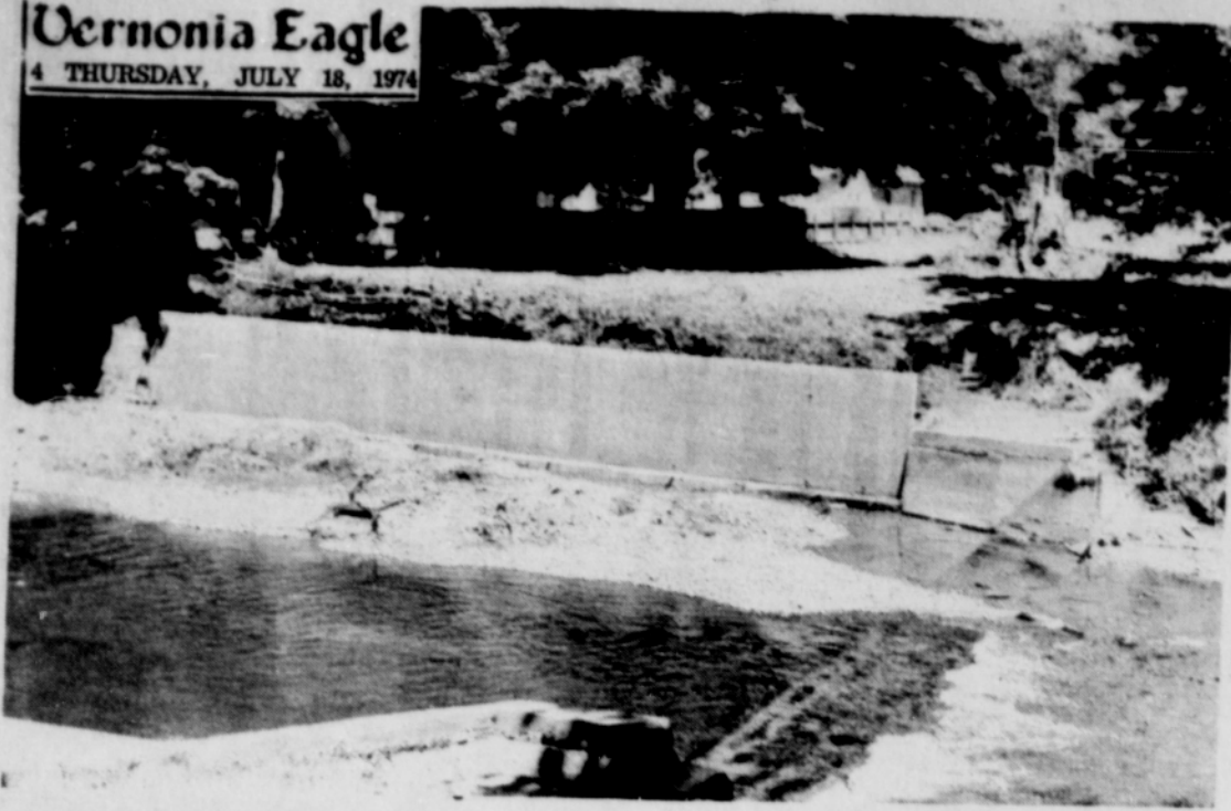
WORK ON the retaining wall continues with the new cement wall now curing—with hopes high that the dam can be put in place at the swimming pool sometime in the very near future.
