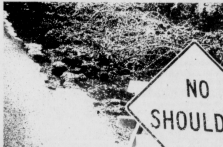
FURTHER signs of water damage to roads are seen in the Riverview area as testified by this sign "No Shoulder." Roads throughout the county suffered similar damage with estimates for repairing the area highways and other destruction running in the $500,000 bracket.
