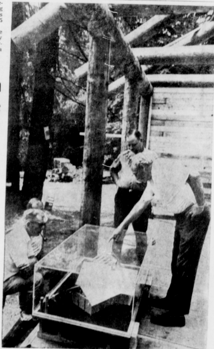
BUILDERS Mel Harper of St. Helens (left) and Leonard Anderson, former St. Helens resident, confer with Commissioner A. J. Ahlborn as to "Where do we go from here?" The Wilkerson Lodge building is ready for the rafters to be framed in on center span, and the builders were called in to plan an attack on the job. A number of volunteers will be sorely needed the next couple of weeks to accomplish the chore.
