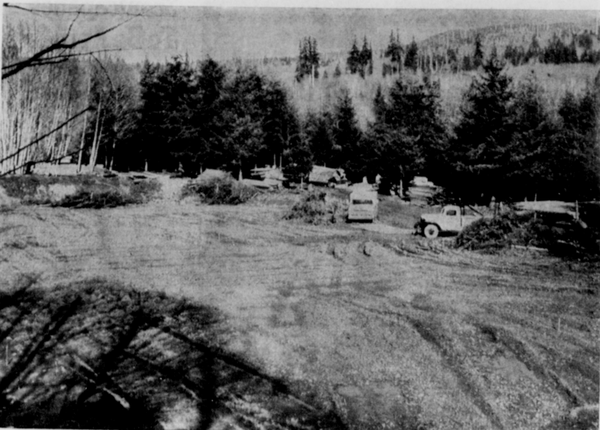
CLEARED area is location where tennis and basketball courts will be built at Sports Acres boys camp near Jewell. Buildings to provide living facilities for boys will be built along line of trees in background.
