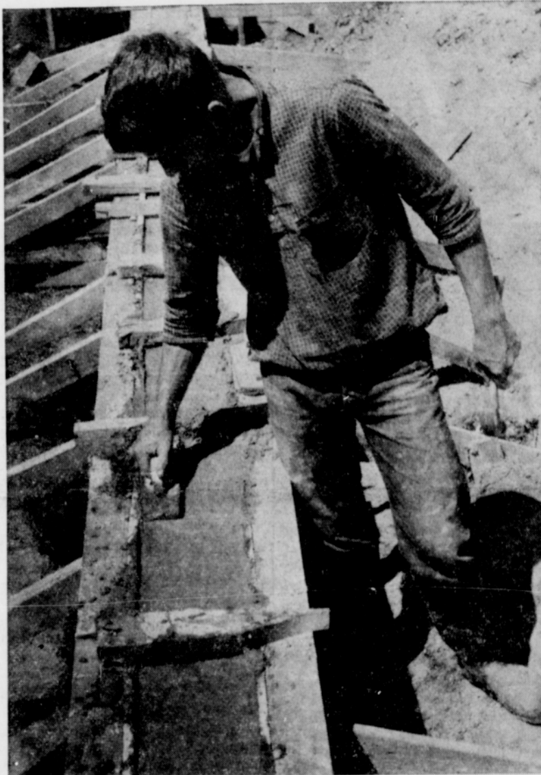
LARRY OBLACK, above, is one of the FFA members busy on the work-type project in which members get practical on the job experience building an addition to the high school shop. Here he works on the concrete foundation.
