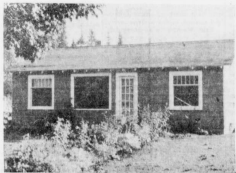
BILL CARMICHAEL enlarged the front of his home six feet, making possible addition of one room and enlarging of two other rooms. He also poured new foundation and installed larger front windows and sided house with composition shingles.
