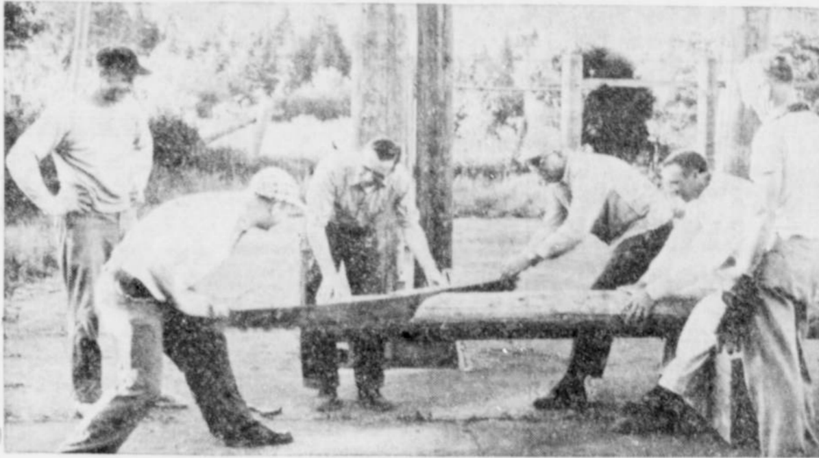
LIONS CLUB members have been working every Monday evening since early in May on their current project, a community kitchen at the city park. This crew was busy framing the structure, part of the poles having already been placed as seen back of the men. From left: Lion President Bill Vicek, Jim Davies, Tom Bateman, Glen Hawkins, Kerry Moran and Cecil Johnson. Several more Monday work evenings will be necessary to complete the project. Hawkins is supervising work.
