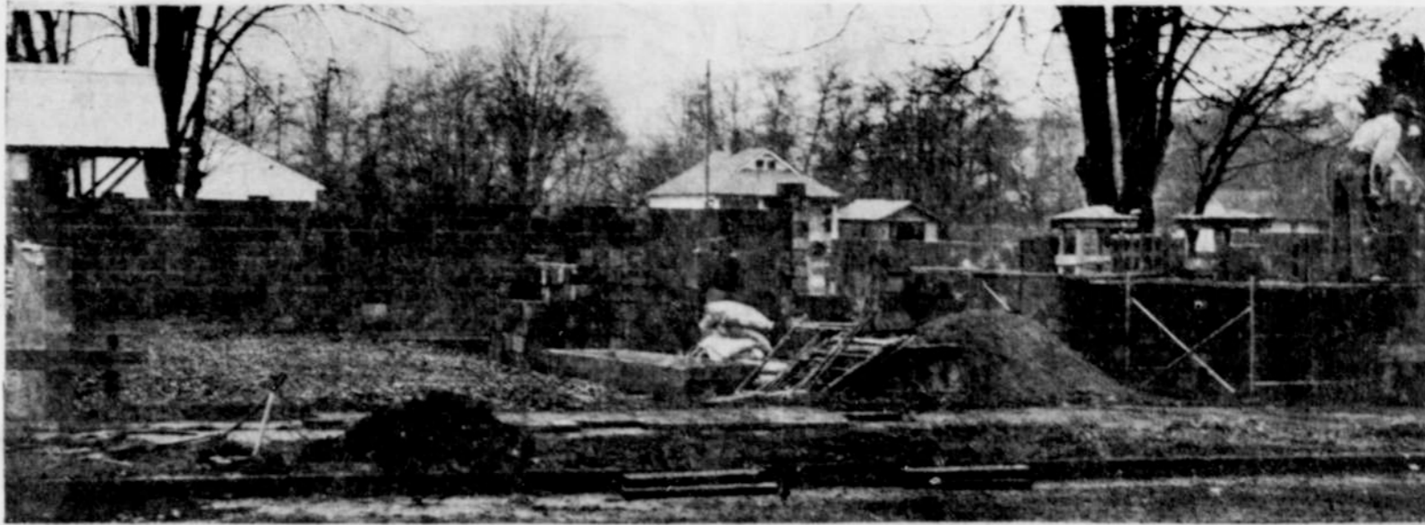
WORKMEN had part of the walls up on the new post office building at Second and Maple when this photo was taken recently. The building will be 46 feet by 44 feet eight inches and will provide 1611
