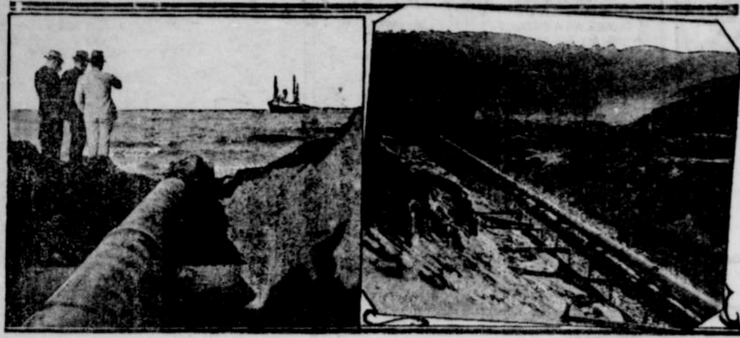
The photos cover incidental features of the actual laying of an ocean pipe line, which was towed to sea by the steamer "Peacock," which is seen in the distance, after having been welded into a single piece on shore. A cable line was made fast to the nose of the pipe line by a special bridge. The pipe line rested on a long runway, which was heavily greased. Skids under the pipe gave the pipe its half mile "ride" down to disappear in the ocean, and were cut away as the pipeline slid into the water. The operation was engineered by the General Petroleum Corporation.
