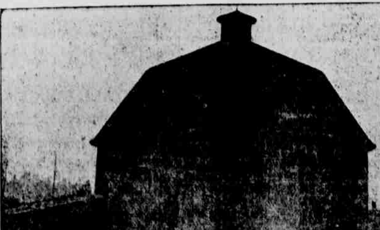
A Combination Barn and Silo, being built by Clarence Alden, near Tillamook. The Silo is situated in the center of the Barn.
