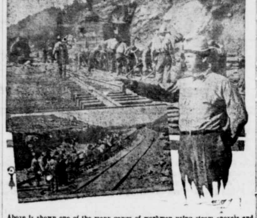
Above is shown one of the many gangs of workmen using steam shovels and other equipment to open the way through the famous Emigrant Gap for additional trackage. (Below) Track laying crew setting a fast stride between Montello and Leray in Nevada. Engineer Ods Weeks directing important construction work.
