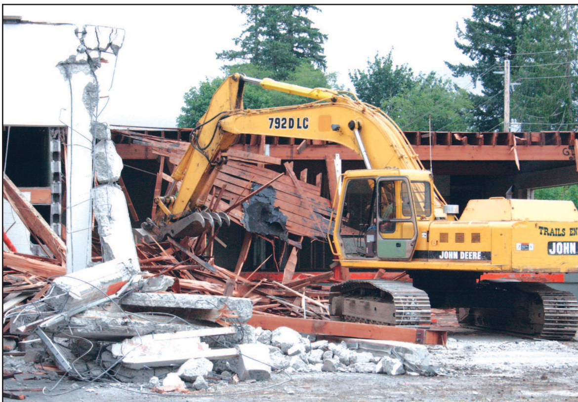
This is what the old West Oregon Electric Co-operative building looked like last week as the demolition continued. See article on this page for information on flood recovery projects.
