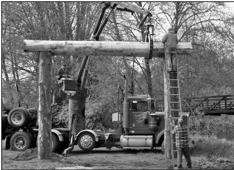
On April 27, Steve Weller brought his self loader log truck to Anderson Park to help the Ridge Riders put up a new entrance to the horse arena. Joe Chestnut is on top of the ladder getting ready to hammer in a stake, and Richard Meyer is holding the ladder.
