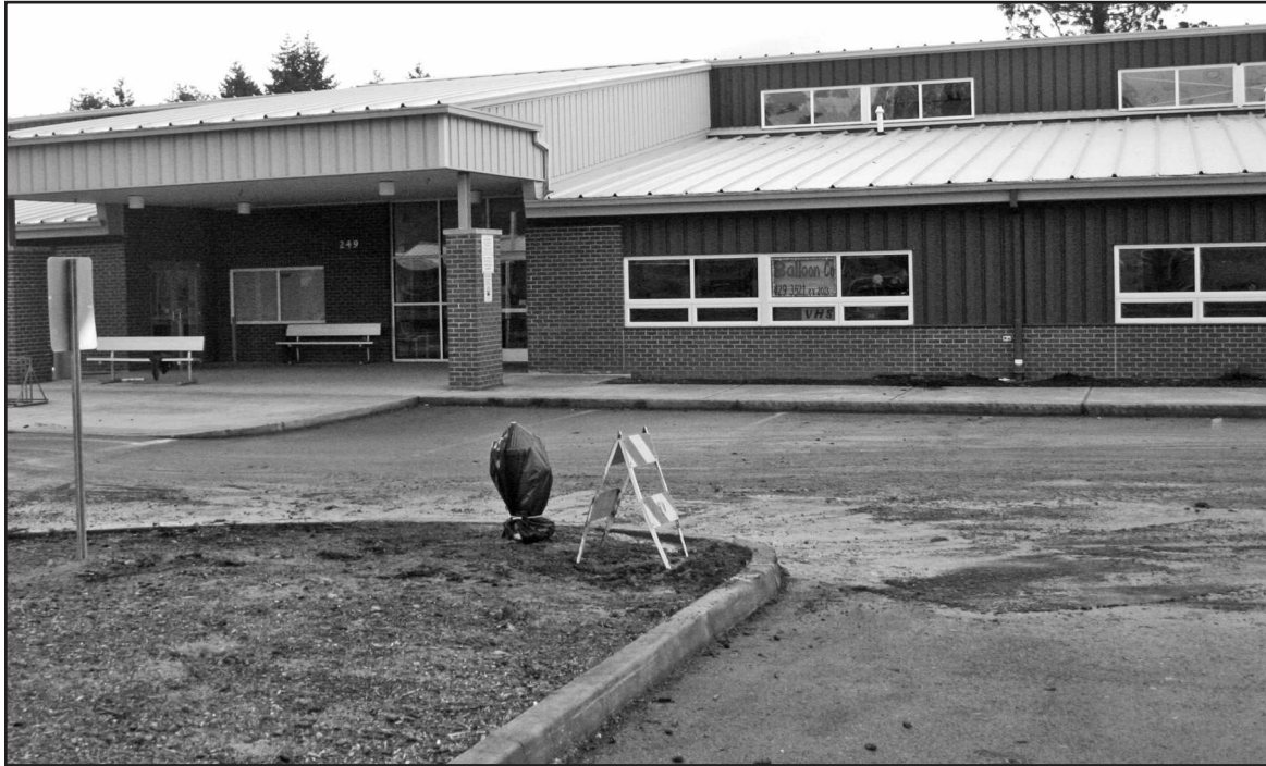
This was the scene Monday morning when school should have resumed after Spring break. Damage to this fire hydrant kept school closed for one more day.
