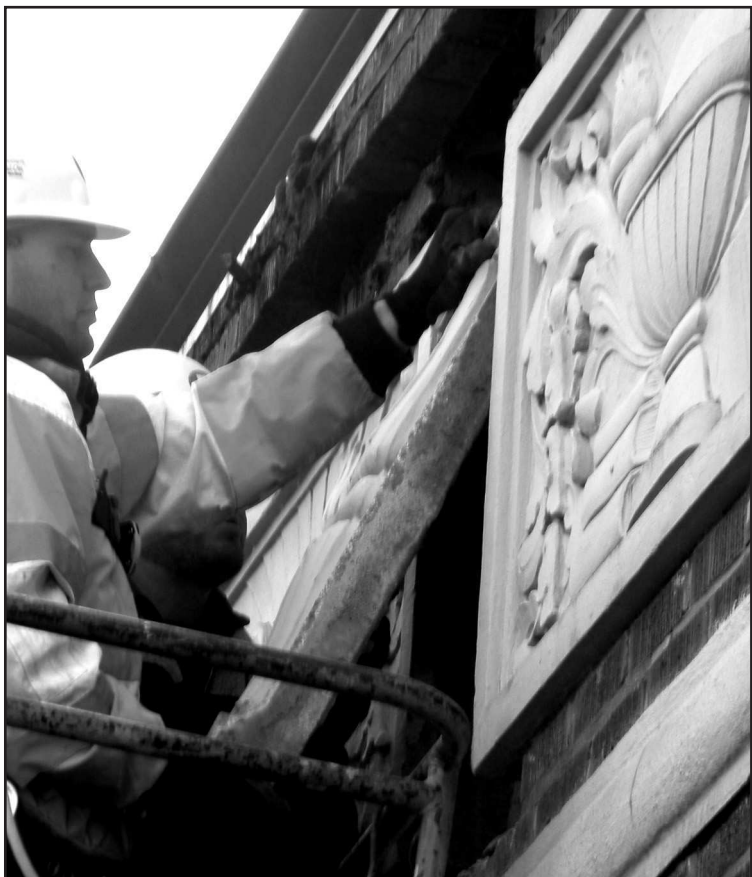
A piece of masonry was removed this week to determine its weight. New Spencer Park will include a historical monument to Washington Grade School. See Chalk Talk above. Photo courtesy of Vernonia Schools.
