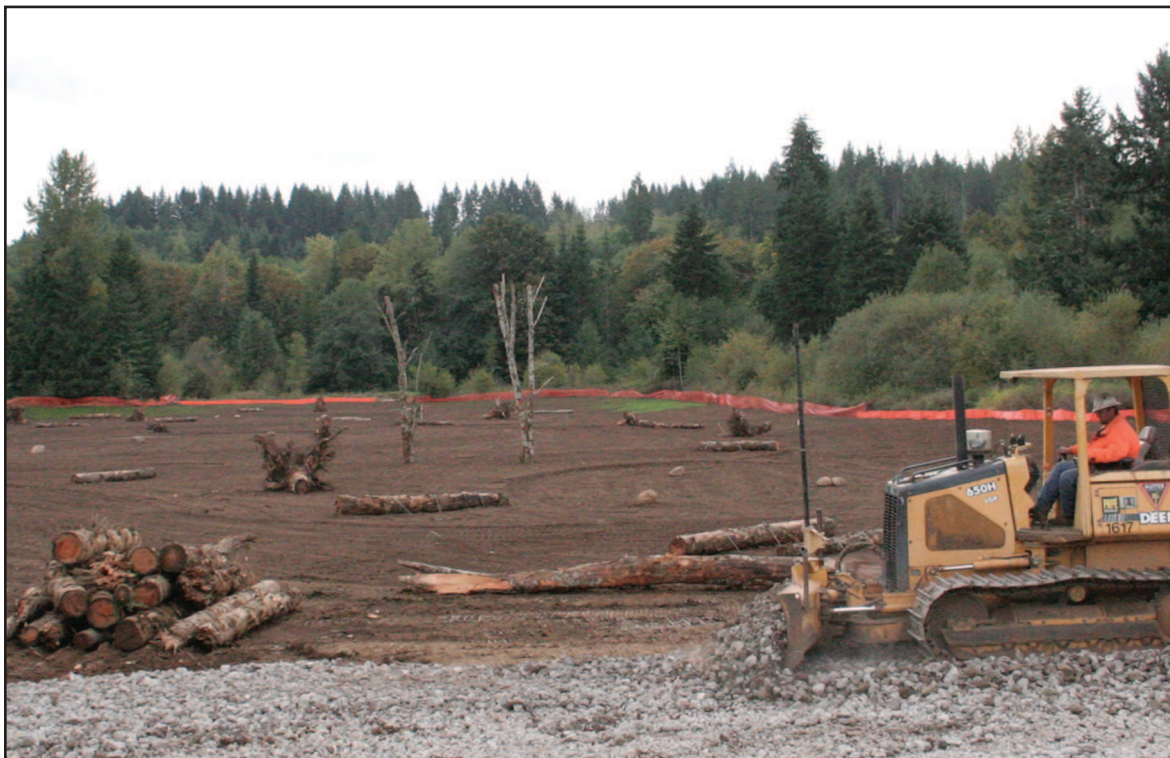
The new wetland, located on the O-A Mill site, is taking its final shape as the excavation work finishes up in the next week. The logs in the middle are being put in place for fish to eventually hang around. See full story on this page.
