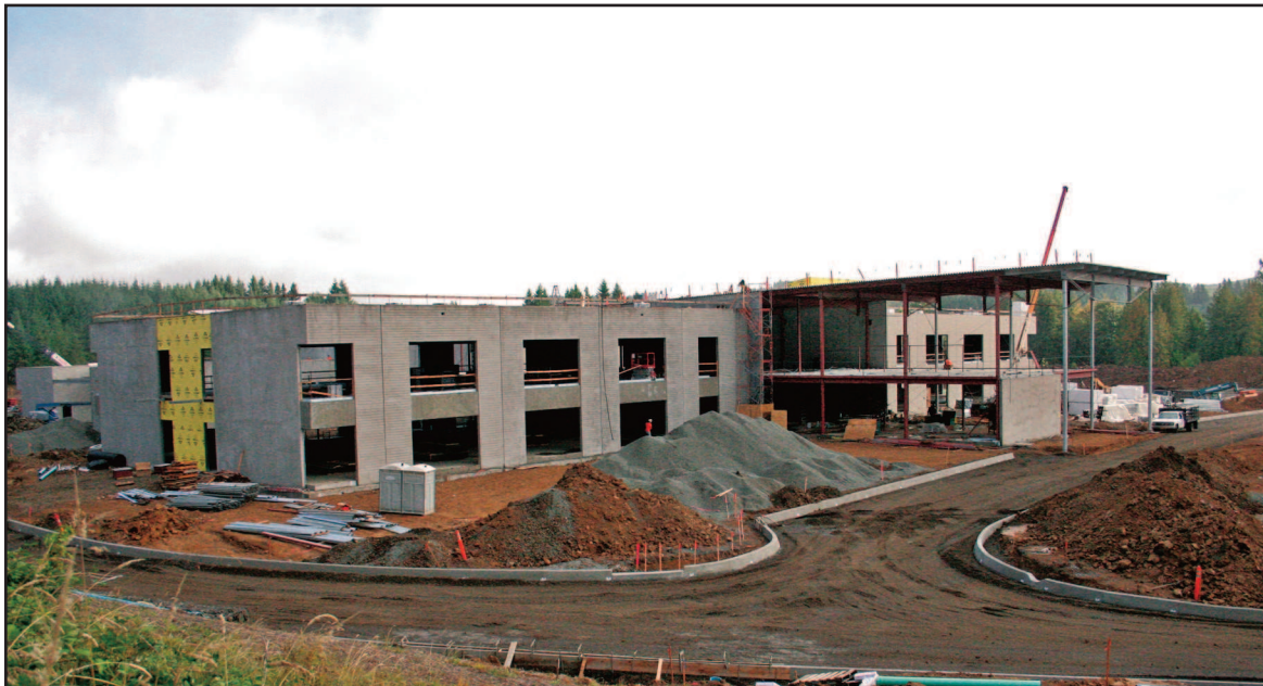
This picture of the new Vernonia school was taken on September 19 and shows the ongoing progress as the builders prepare to finish the roof before the winter weather sets in.
