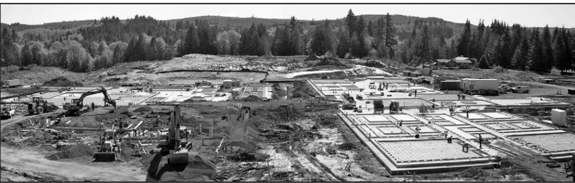
The new school site, as seen on May 18. Concrete is being laid and the project is on schedule, but obviously has a long way to go before the doors open.
