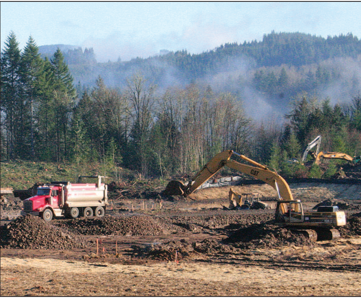
Despite recent heavy rains, groundwork on the new school construction is on schedule. Construction on the building is scheduled to begin March 1.
