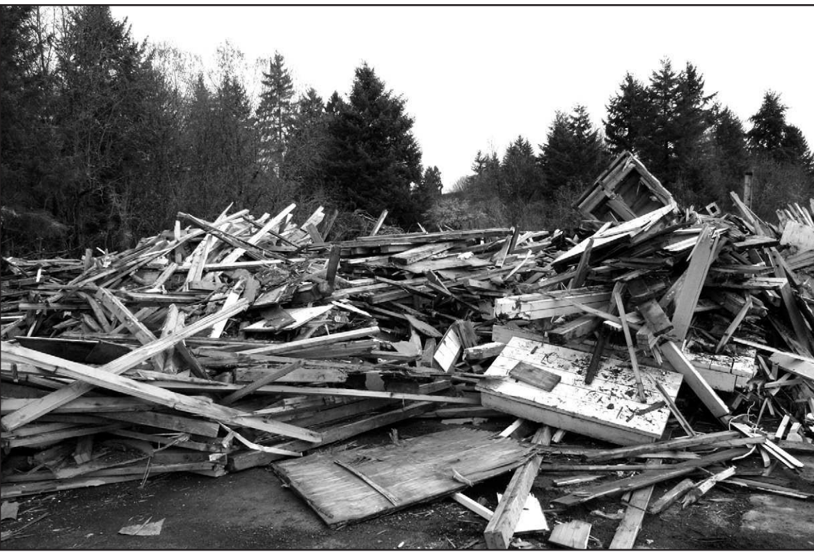
The debris from the houses being demolished, due to flood damage from 2007, is being staged at the old mill site. Parts are being recycled and part will end up in landfills. This pile represents three homes of the four currently contracted for demolition. Five more are pending demolition and 13 homes have been elevated. Two homes are currently being elevated.
