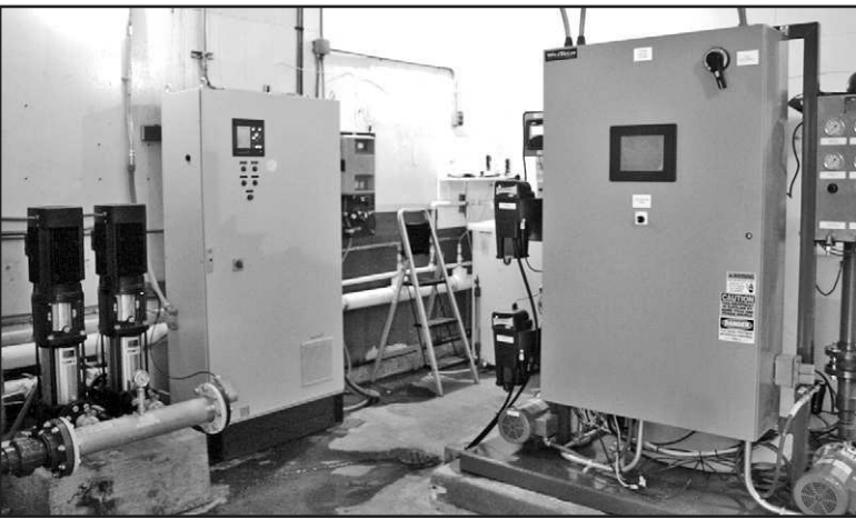
A peek inside the new water plant in Timber shows the pumps on the left with their computer beside them and the new membrane treatment component on the right.
