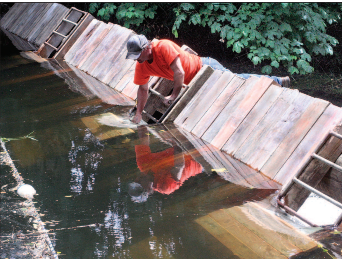
Summer is here now that the dam has been installed on Vernonia's free flowing Rock Creek Swimmin' Hole. Jeff Burch and the Public Works crew said "Come on in, the water's fine!"
