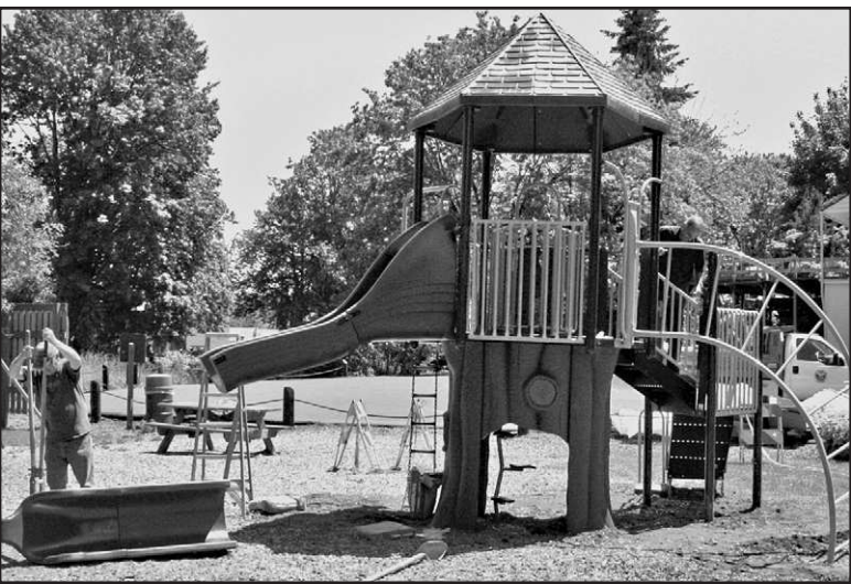
The Vernonia Parks Committee recently purchased new playground equipment for Hawkins Park. On June 16, Public Works employees, Carl Pense and Jim Gido, were installing the new equipment. It should be ready for the kids by now.
