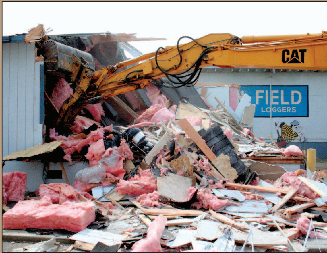
The removal of Vernonia School District's water-damaged modular classrooms is one of many jobs made necessary by last December's flood.
